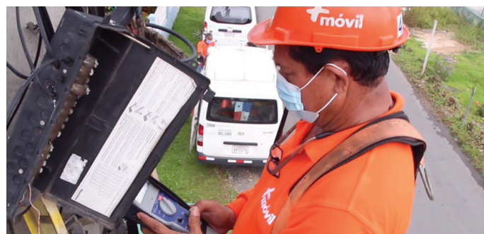
Our Cable & Wireless Panama technician in the field working to keep our communities connected
