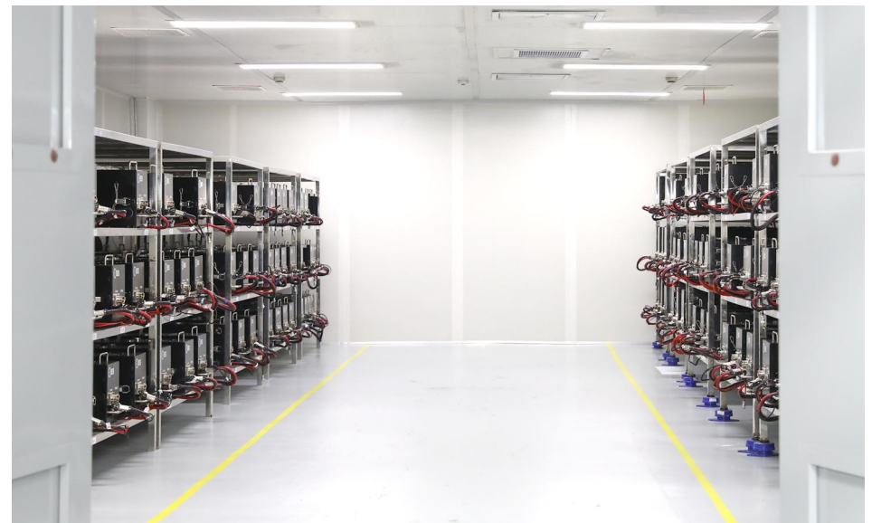
Test bunker for automotive Li-Metal cells
